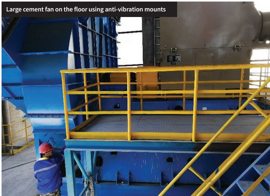
A large steelworks fan on a concrete foundation
