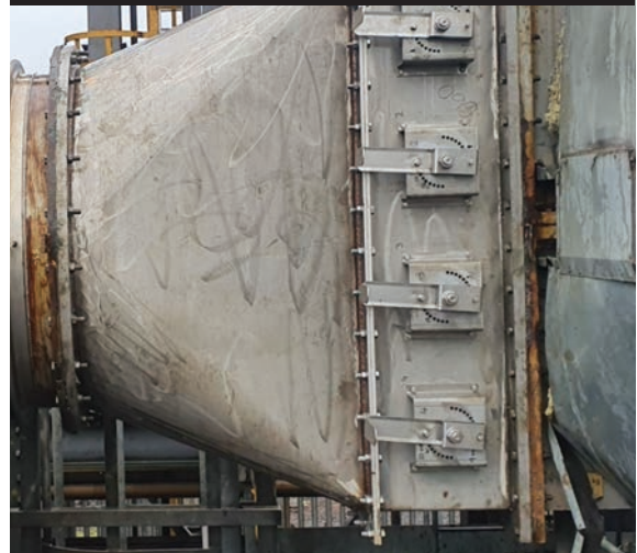
Manual box damper retrofitted on centrifugal fan – used to match fan VSD performance to system curve
