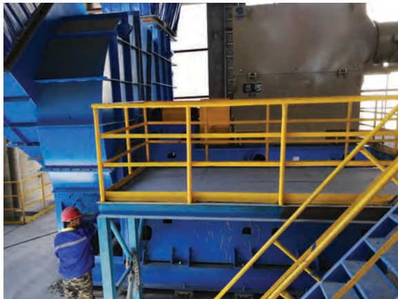
Large cement fan on floor close to process using anti-vibration mounts.
