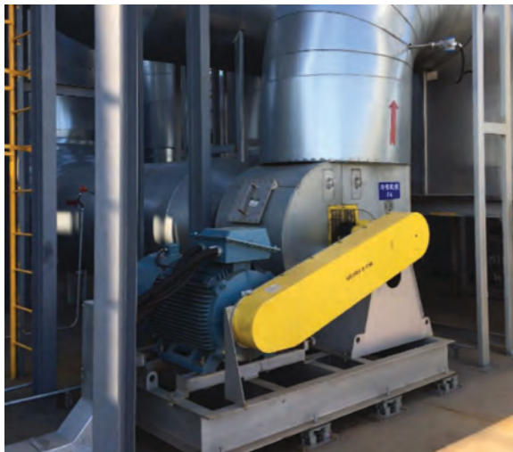
Belt-driven fan on anti-vibration mounts.
