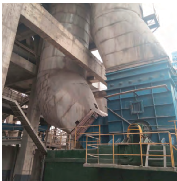
Large cement fan at ground level. Ducts rising to process using anti-vibration mounts.
